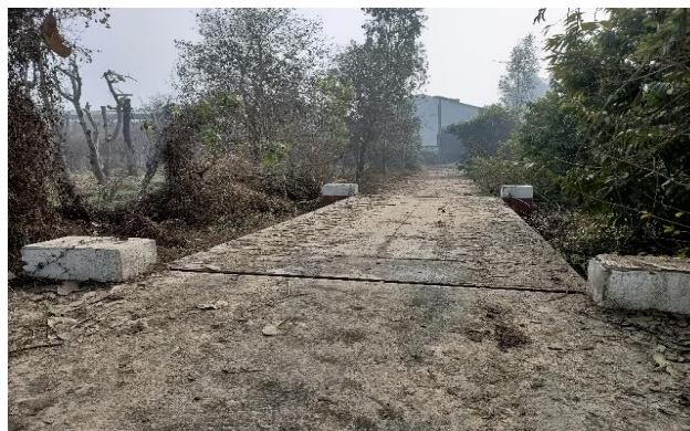
Figure 44 Abandoned approach in Rajau Paraspur SWM Plant
