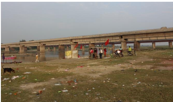
Image 49: Dilapidated Ghat along river edge and connecting bridge
